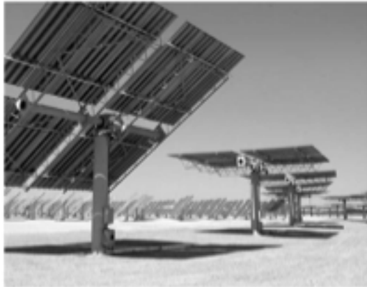
FIGURE 3.22 Detail of a heliostat.
