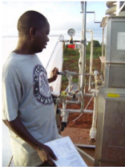
Figure 11. The system is operated by manual valves. Operation is routine and easy to do. The valves are operated in the morning and late afternoon. Water to be frozen is put into the evaporator in the afternoon; it is ready to be removed as ice early the next morning.
