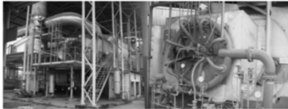
Fig. 2. View of the Barreiro power plant boiler (left photo) and detail view of the fuel feeding system in the boiler (right photo), with the central hole (open tube) used for wood tar injection, and the main round tube used for steel furnace gas injection.
