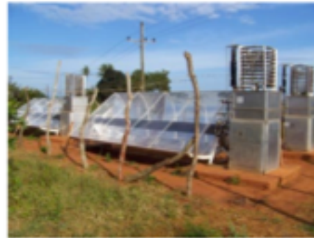
Figure 3. Three units were installed in Kilifi District at Sovimwamri Dairy.
